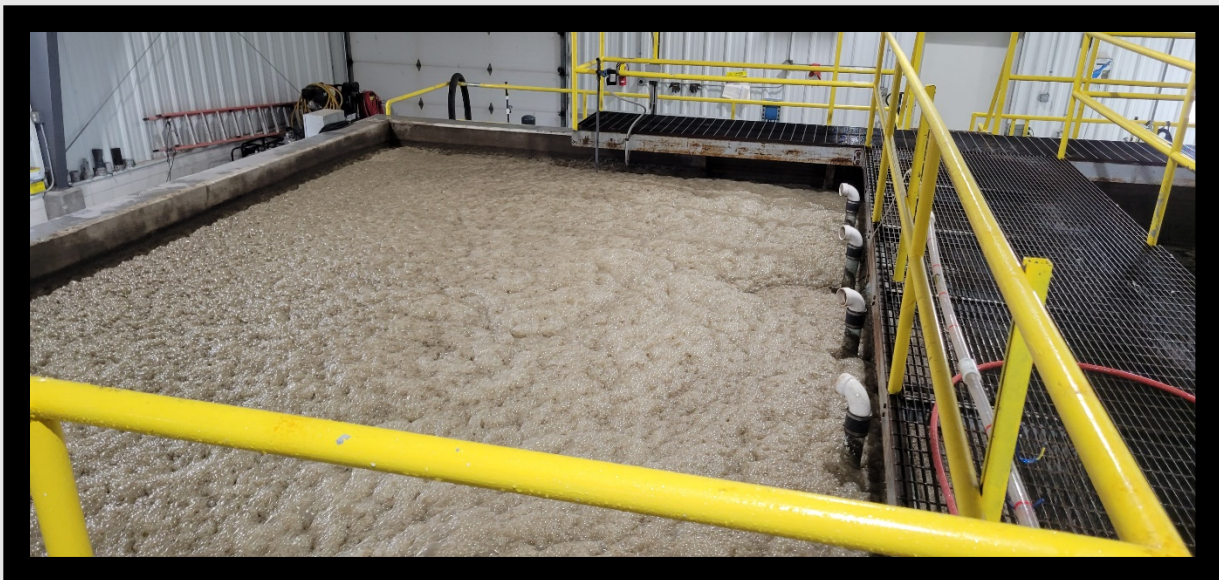
Foam on the aeration basin at Aspen WWTP 4/25/22.
