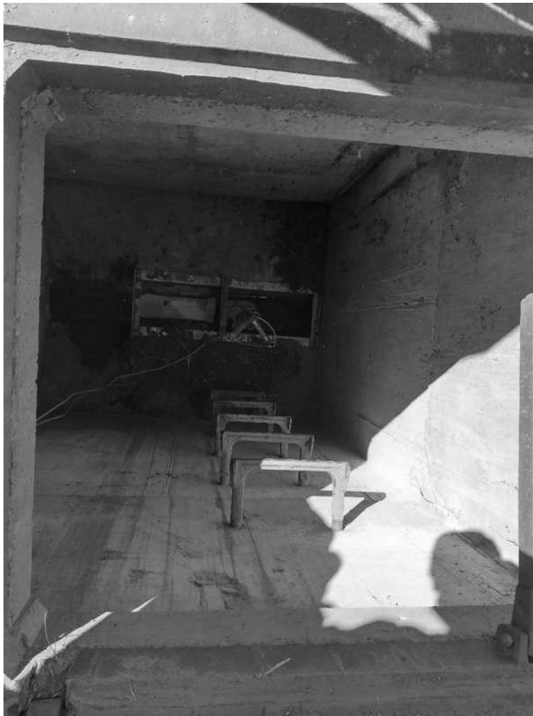
Figure 1 – BGWSD / Crestone Wastewater Master Meter
