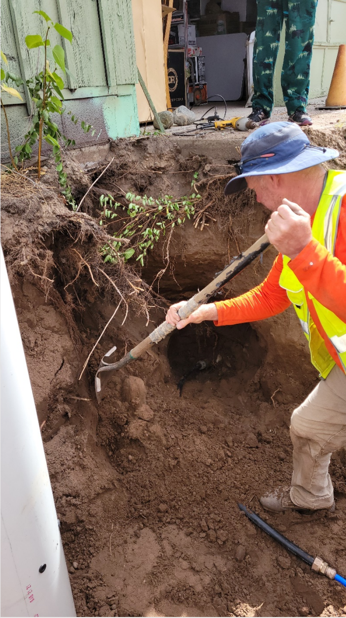
Picture showing water main under garage.
