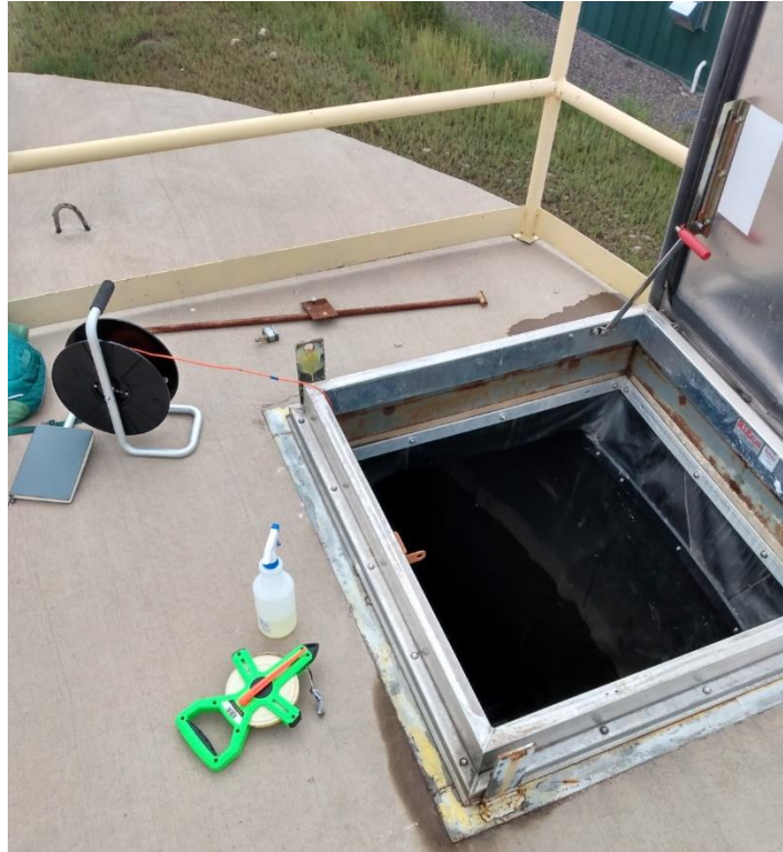
Figure 3: Well 18 Tank Opening
