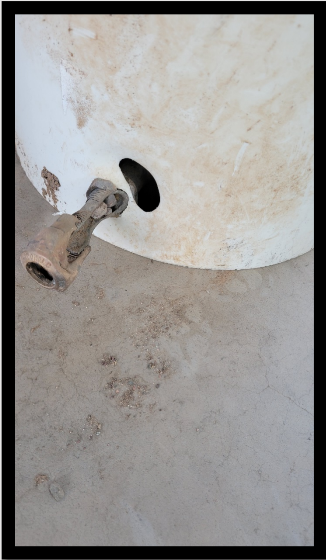
Water erosion of Meter pit in less than 24hrs.
