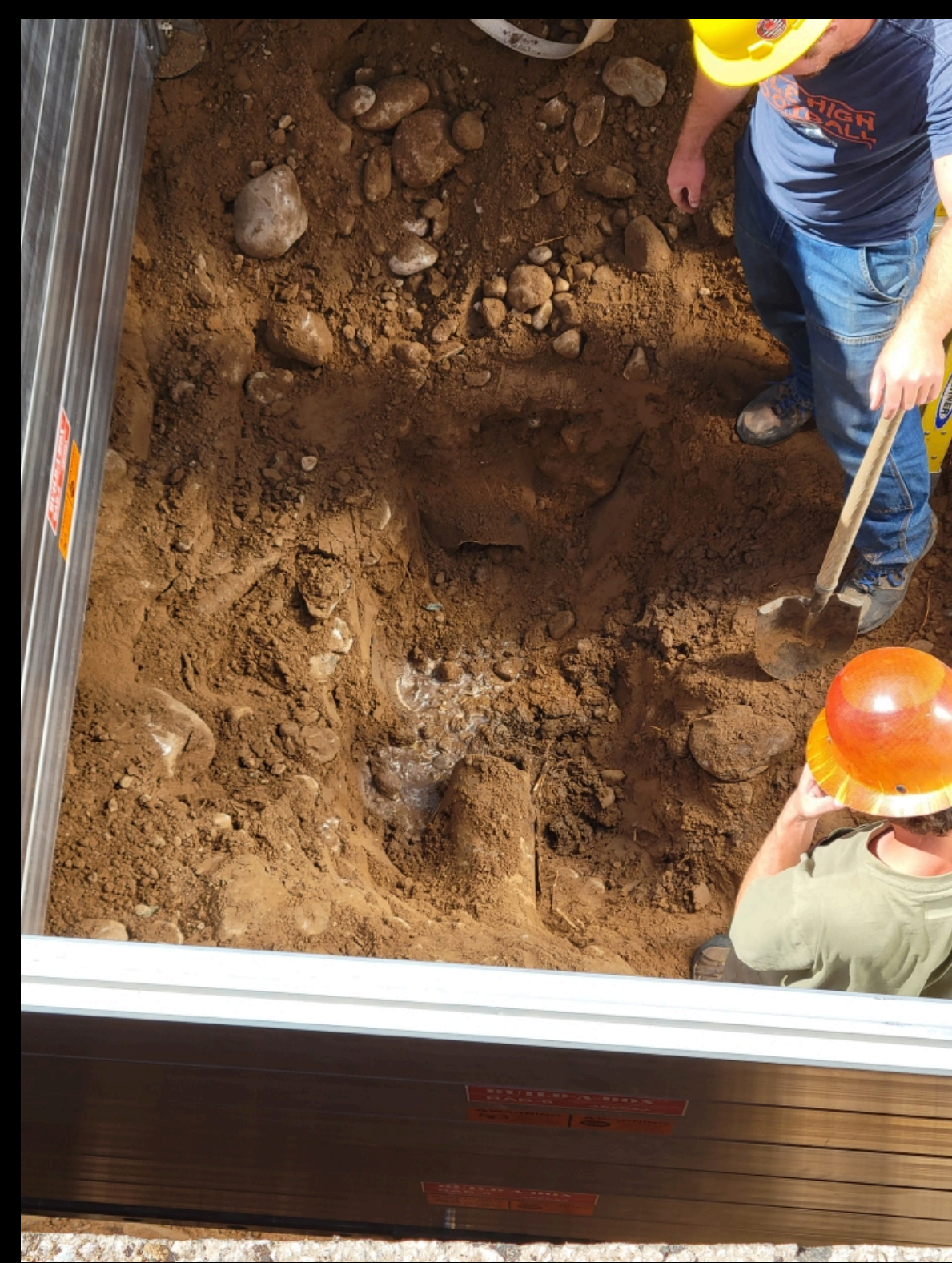
Sewer Main Line On Camino Del Rey before repair.
