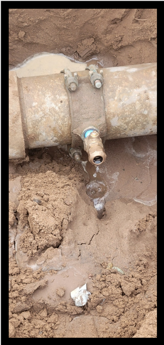
Leaking Curb Stop on AC Water main in Casita Park
